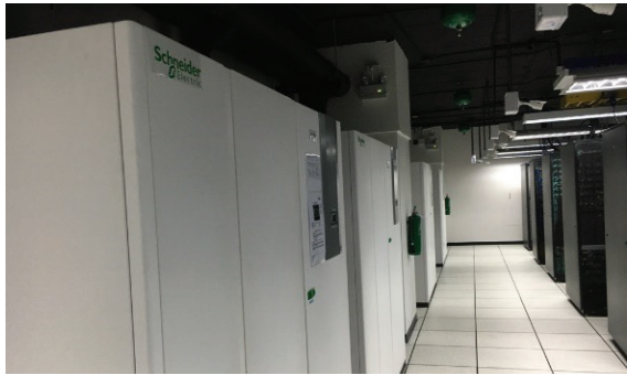
Data Center area of PROEN at NT Bangrak Building
